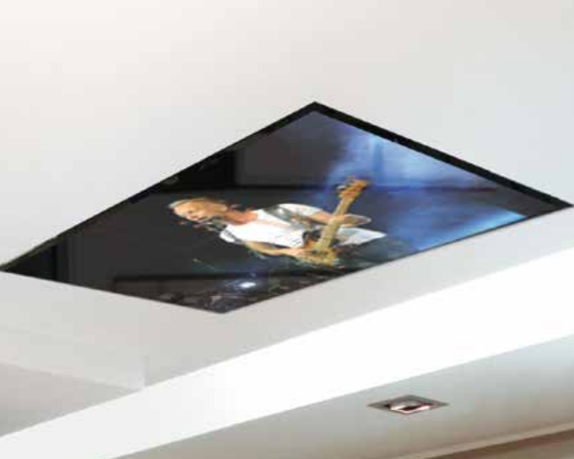
Screen flush with the ceiling
